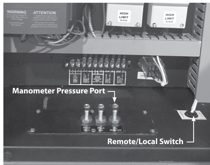
Figure 22 Manometer connections to manifold
